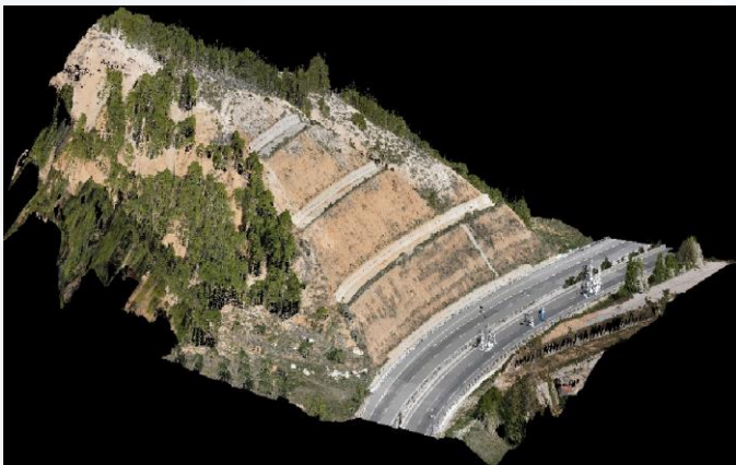
Figure 5: Example of point cloud of a slope in Spanish A2 motorway generated after processing with photogrammetric techniques.
